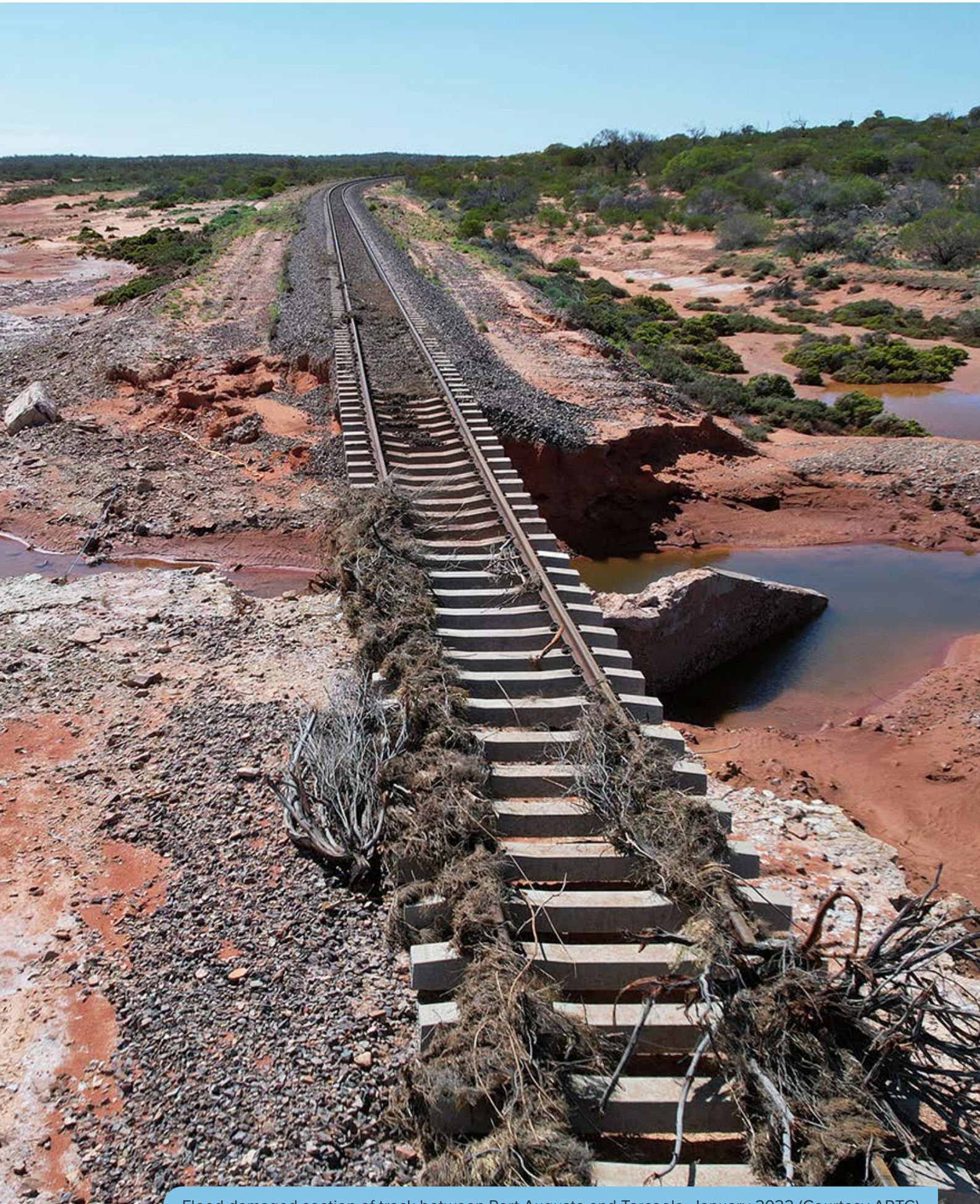
Flood damaged section of track between Port Augusta and Tarcoola, January 2022 (Courtesy ARTC)
