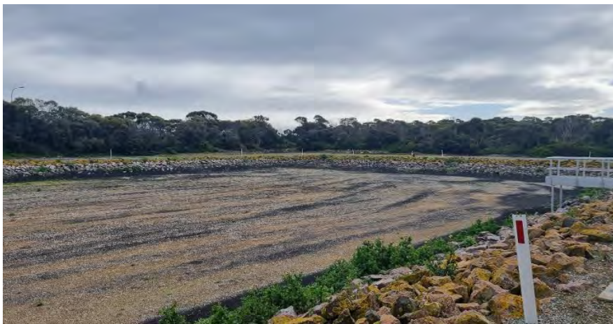
Figure 7.4 Marine intake and outfall pump station site in disused lagoon at the WWTP
