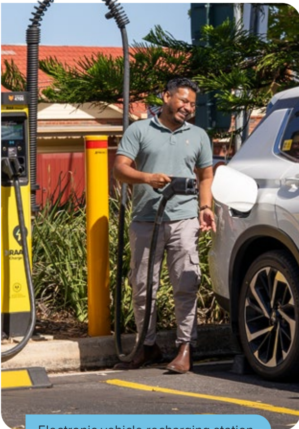
Electronic vehicle recharging station
