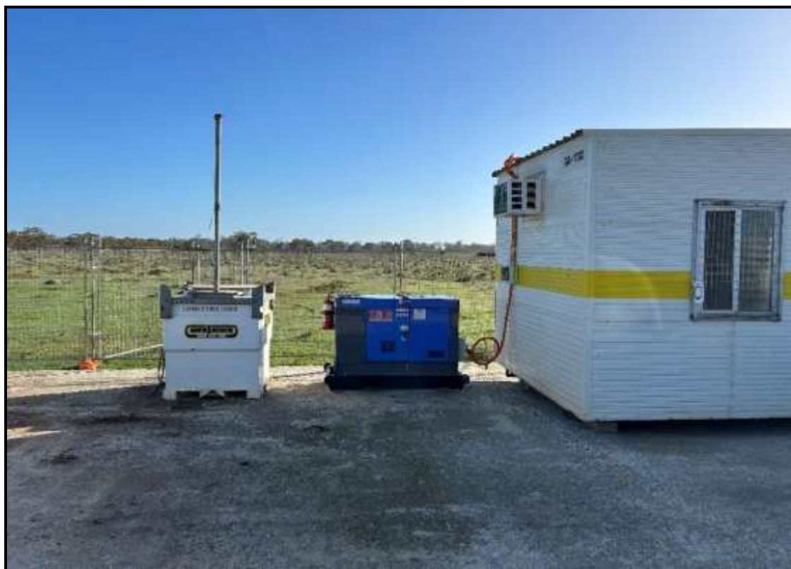
Photo 9 – The 990 L self-bunded diesel storage tank and generator in the construction compound
