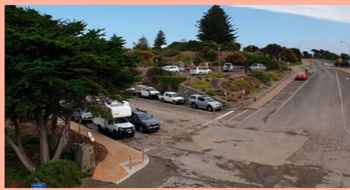
Greening provides buffering and amenity, contrast to damaged road surface
