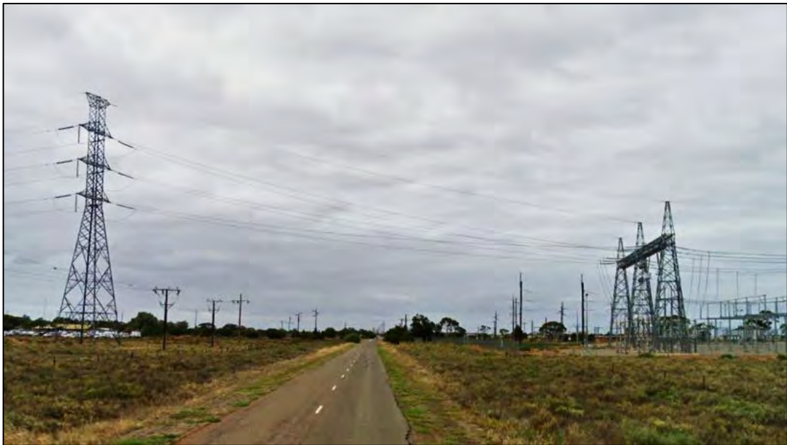
Figure 4-10: Existing Transmission Lines and Tower Connecting to the Bungama Substation
