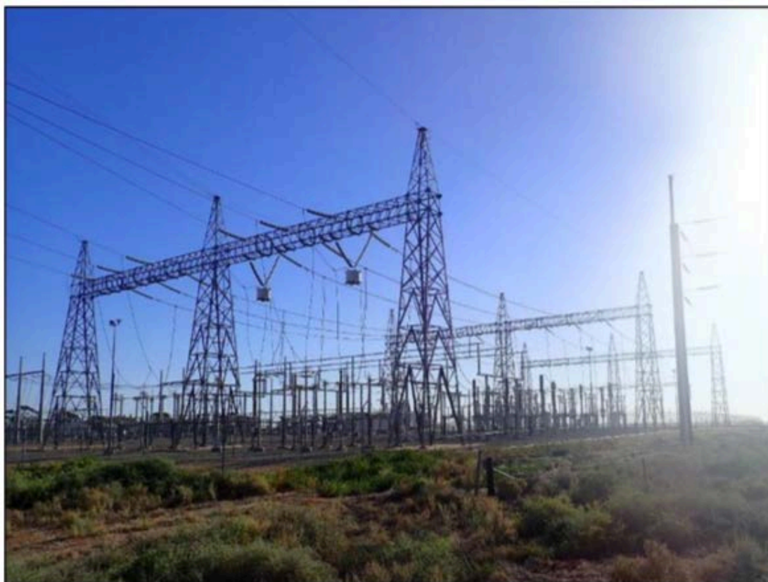
Figure 8 – Bungama Substation (Source: EPS Energy, Nov 2018)
