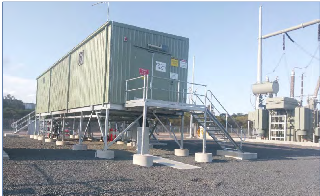
Figure 4-6: Example of a Typical Switch Room
