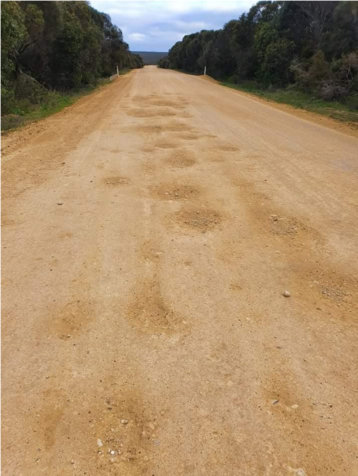
Massive potholes over road
