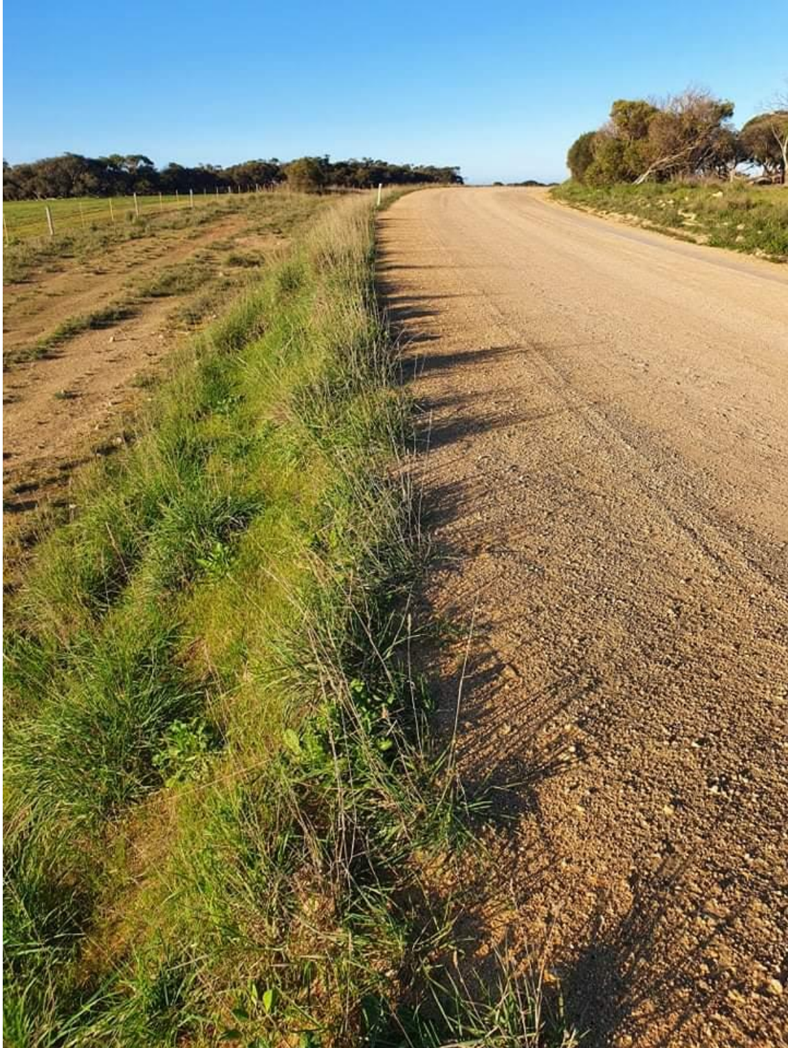
Drop off of several feet on side of narrow corner
