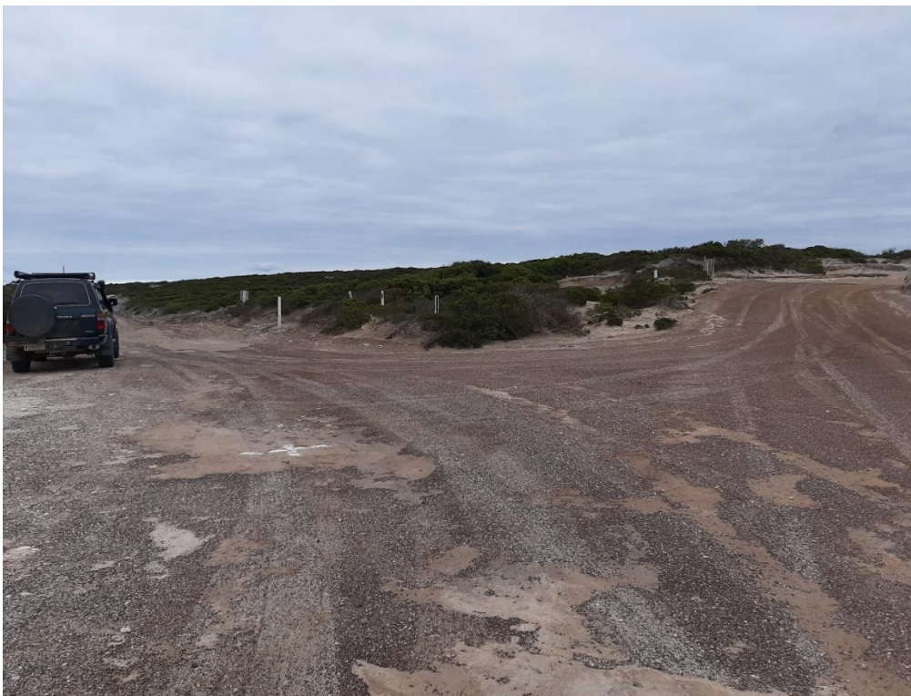
Figure 18 – Access Track Junction Seagull Layout “Cape Wiles” (looking north east). SISD on approach of the junction is poor for the southbound major alignment (<106m) but reasonable for the northbound major alignment. ASD is reasonably good.
