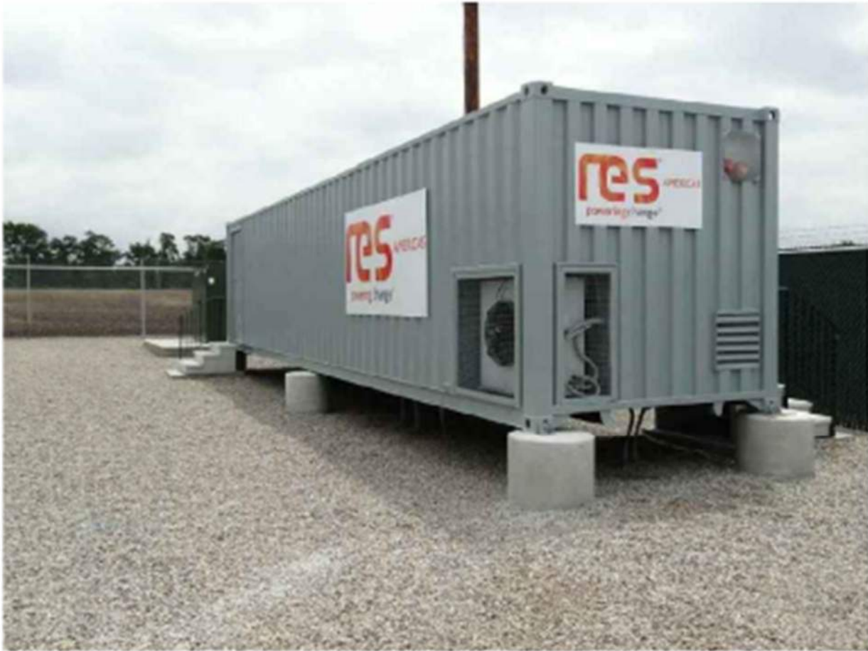
Figure 5: Typical energy storage container
