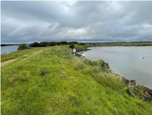
Figure 33: Image of existing levee (view to the east from existing floodgate structure).
