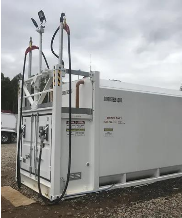
Figure 19: Example of a self-bunded aboveground fuel tank 5
