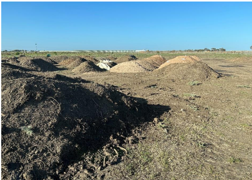
Photograph 5. Stripping of vegetation and topsoil in central portion of Precinct 3A. Surficial soils are being sieved for identification of cultural artefacts. (18.07.2025).
