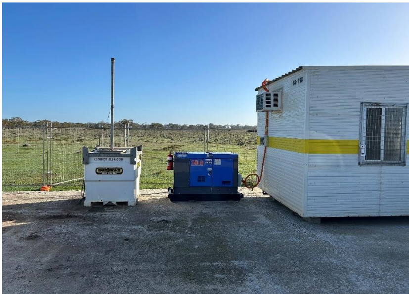
Photograph 8. View to the north of 990 L self-bunded diesel tank and generator in contractor compound. (18.07.2025).
