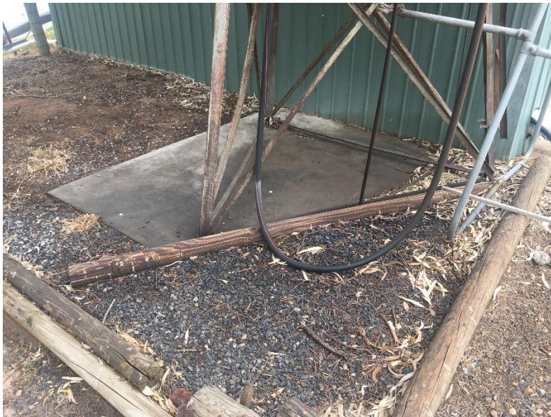
Photograph 12. Surface staining beneath diesel AST on adjacent property to the west. 14.12.2022
