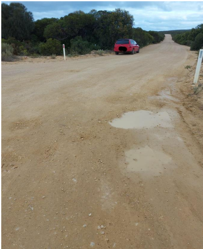
Figures 4 and 5: Large and dangerous pot holes along access road. Many parts of this road are subject to flooding during the rainy season which further exacerbates the instability and erosion.
