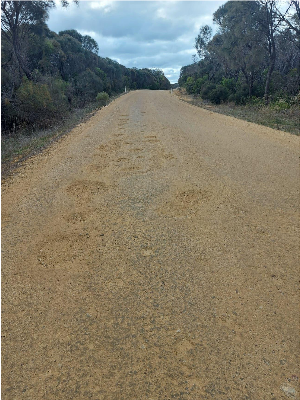
Figure 3: Significant pot holes take up large portions of the access road.
