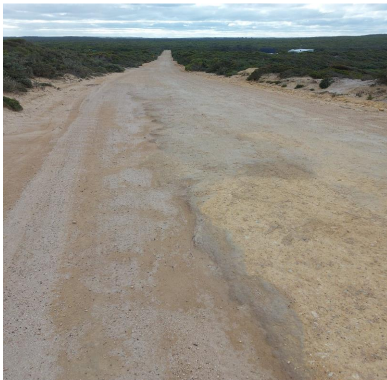
Figures 8, 9 and 10: Areas of significant erosion along access road.
