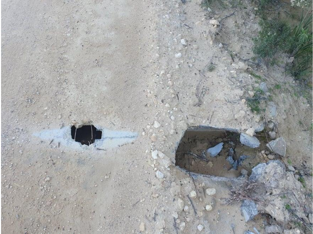
Figure 11: Broken Drainpipe on Fishery Bay Road as a result of increased traffic associated with temporary development.
