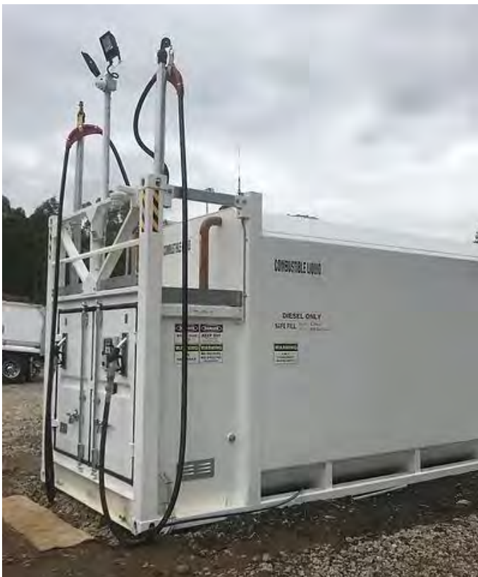
Figure 6: Example of a self-bunded aboveground fuel tank
