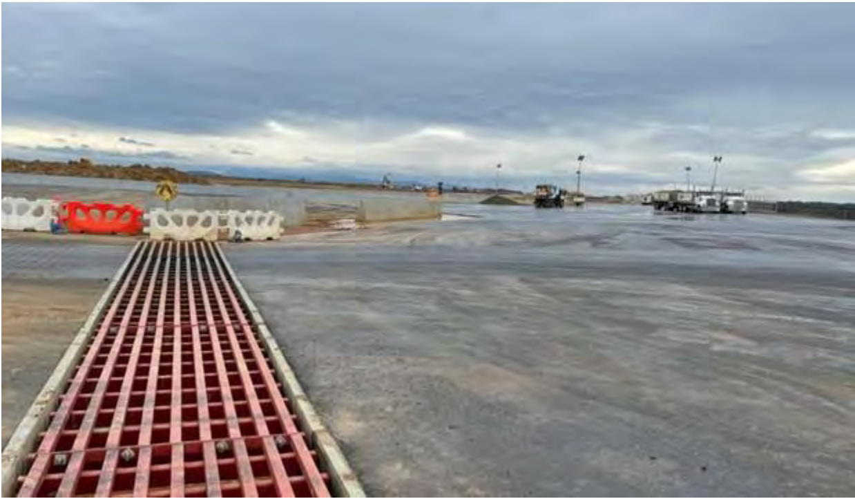
Figure 8: An example of a spoil receival and handling area
