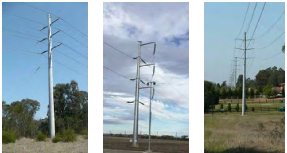
Figure 6: Typical transmission pole infrastructure
