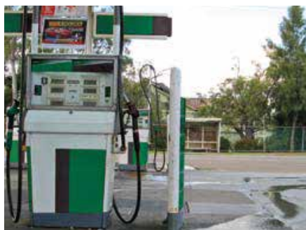
Picture shows a defective forecourt design with oils and fuels discharging directly to the street drain.
