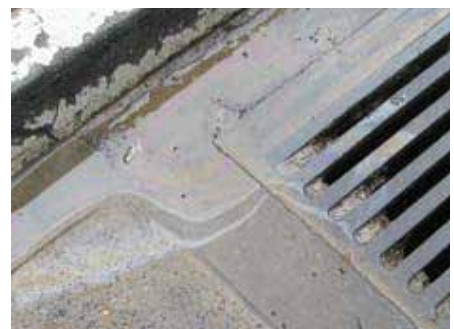
Unseemly & highly visible hydrocarbons polluting the stormwater. The concentration in the picture is in excess of 10ppm
