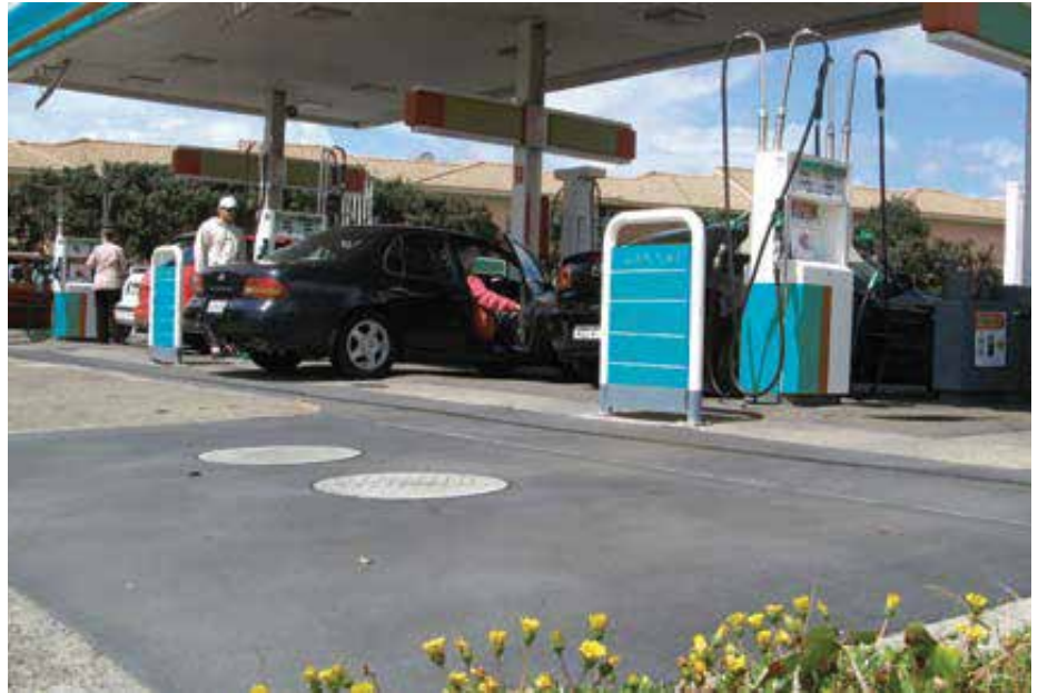
Petrol forecourt and surrounds at a busy metropolitan petrol station rendered compliant. The catchment consists of a grated drain encompassing the complete perimeter of the under-sized canopy. Surface water and forecourt runoff drains to the Puraceptor located under the two trafficable covers in the foreground.
