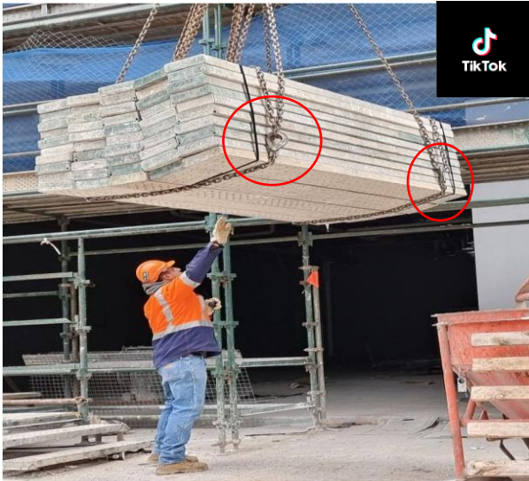
Figure 1- Unsafe rigging practice identified in the industry (Not an ACCIONA workplace)
