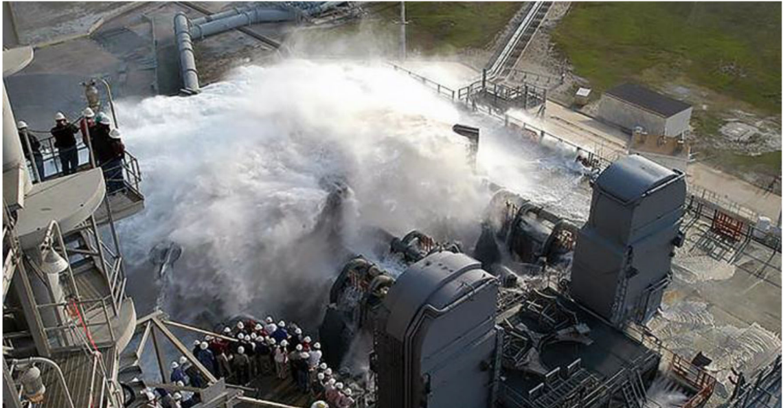
Photograph 8.1: Kennedy Space Centres Launch Pad 39A water sound suppression system. (Source - NASA - https://www.nasa.gov/missions/shuttle/f_watertest.html )
