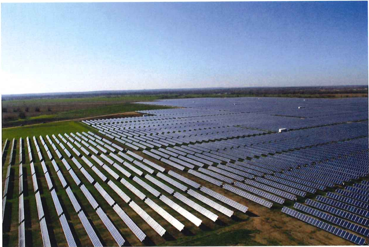
Photograph of a typical single axis tracker photovoltaic panels in a solar farm
