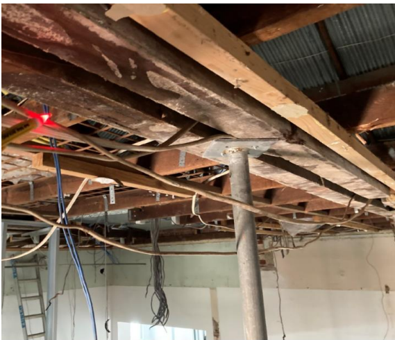
Live existing cables hanging loose in a dangerous state near props and ladders after demolition.
