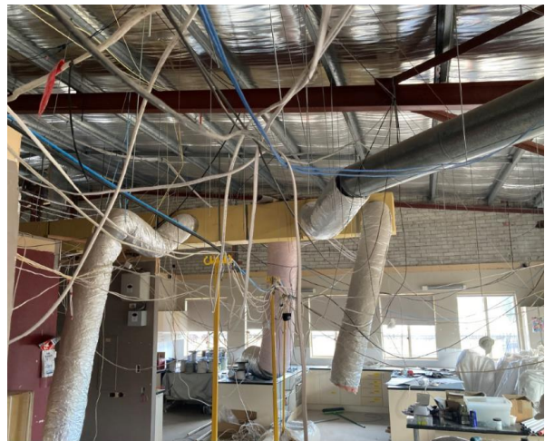
A 'bird's nest' of existing live cables after a ceiling demolition.
