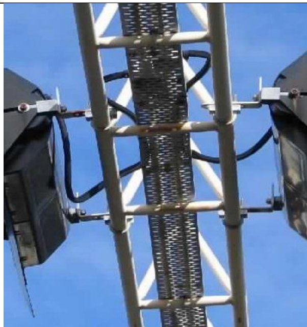
Rust spots on underside of truss members
