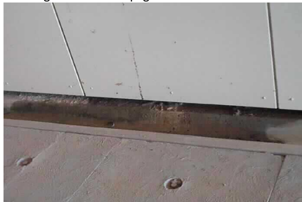
Water in side spoon drain, likely from leaking shrinkage cracks in wall
