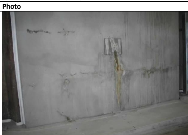
Cracking and water seepage in tunnel wall
