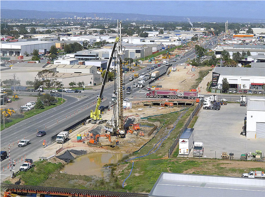
Piling rig operating within the North Arm West drain, an area identified as having a high probability of acid sulfate soil occurrence (ASRIS).
