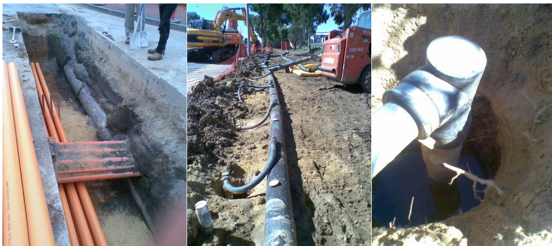
A trench showing newly laid service conduits beneath existing conduits; a groundwater drawdown system for dewatering running parallel to a service trench; close up of one of the spear inlets on the groundwater.
